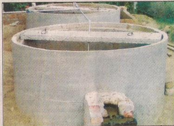
■ The biogas plant
